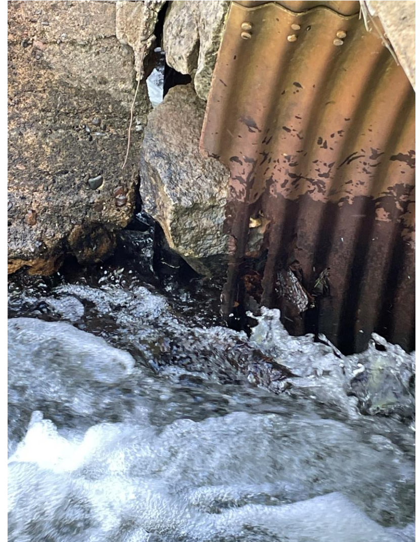
P8: Center pipe deterioration and possible seepage between left and center culvert
