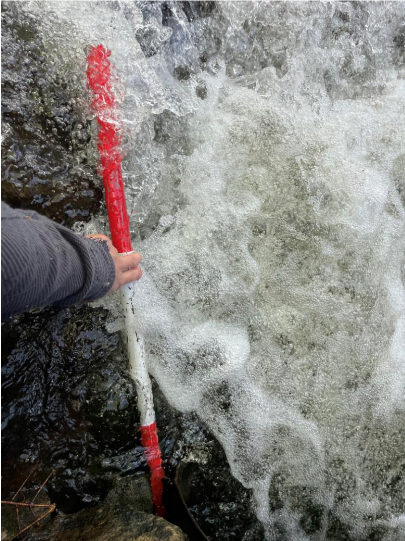
P9: Void along right side of center culvert
