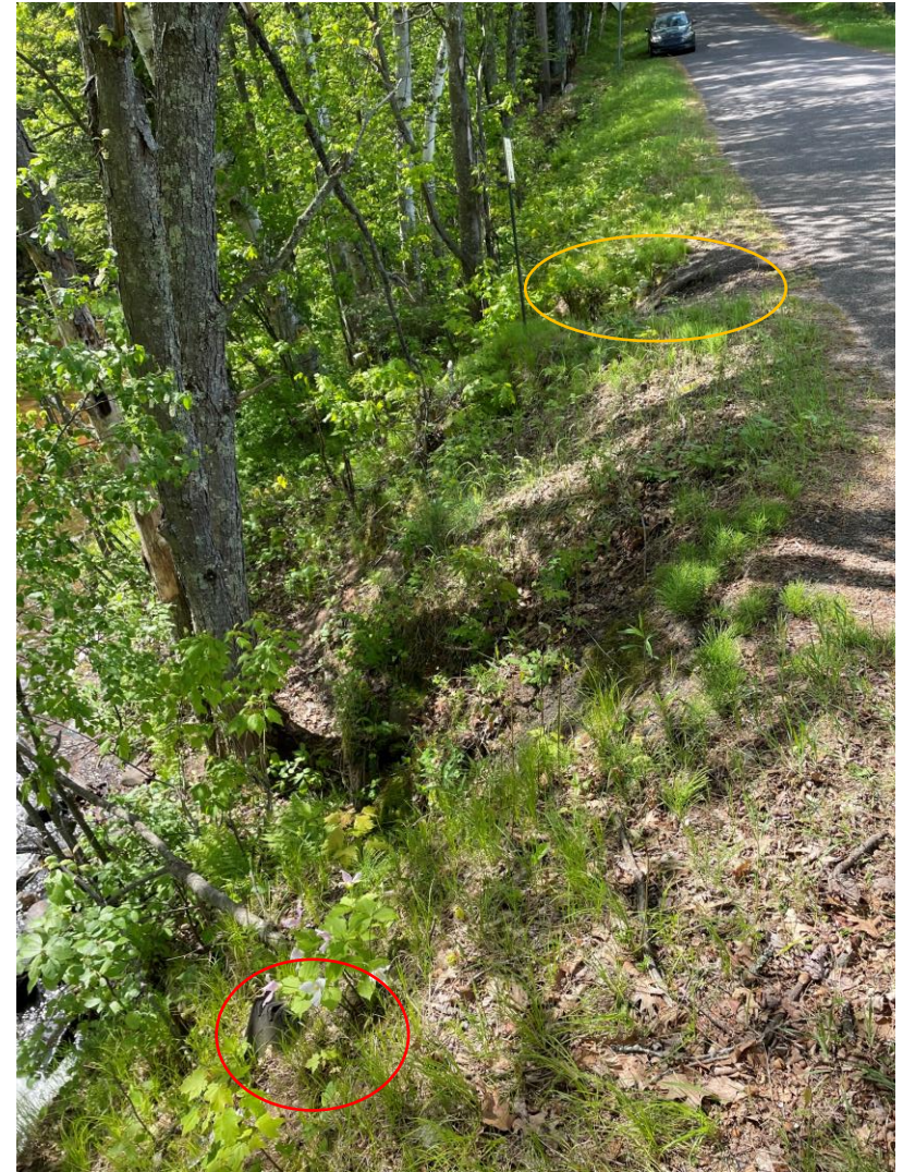
P6: D/S embankment looking right and example of woody vegetation. Tire circled in red. Erosion location circled in orange.
