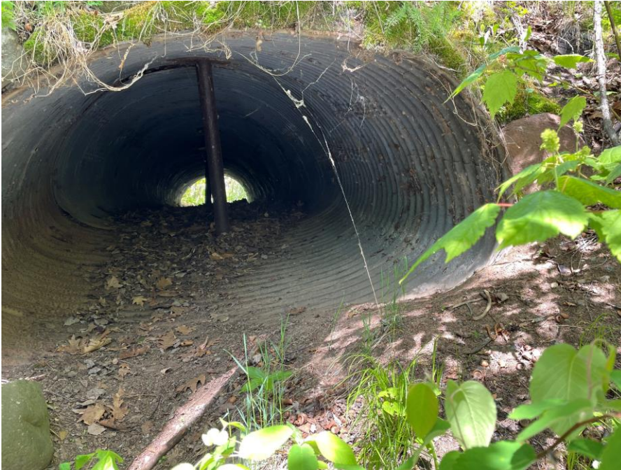
P7: Slumping/deflection right perched culvert looking U/S
